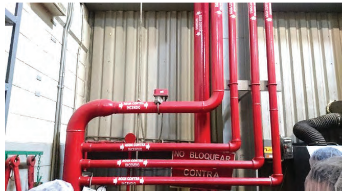
Missing control valve
