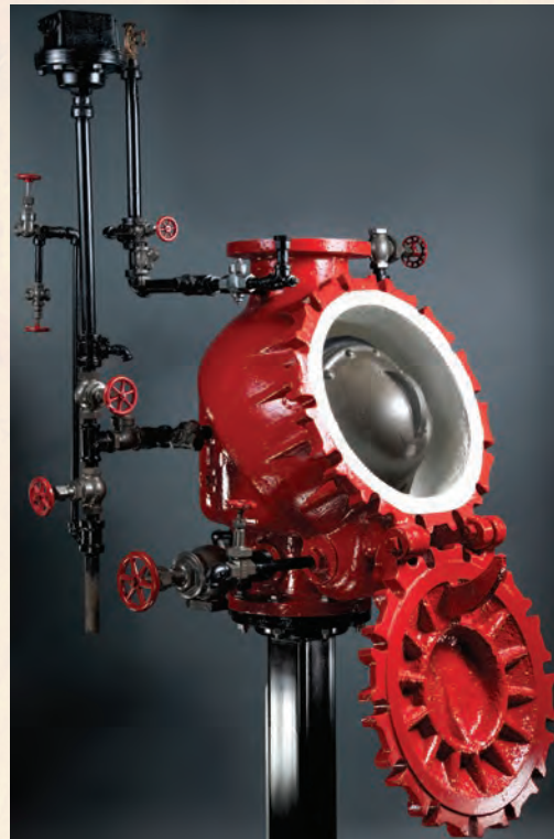
A 1923 Reliable Model B "C" Dry Pipe Valve by the Reliable Automatic Sprinkler Co. Inc. Found still in service in Chicago; it was recovered and restored by millwrights in 2015.
